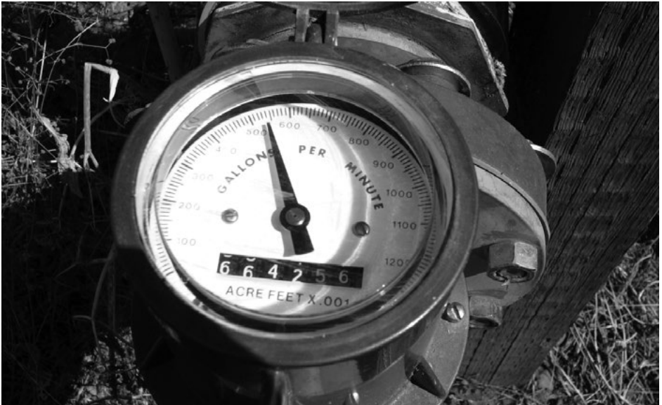
This photo is an example of a water meter device.
